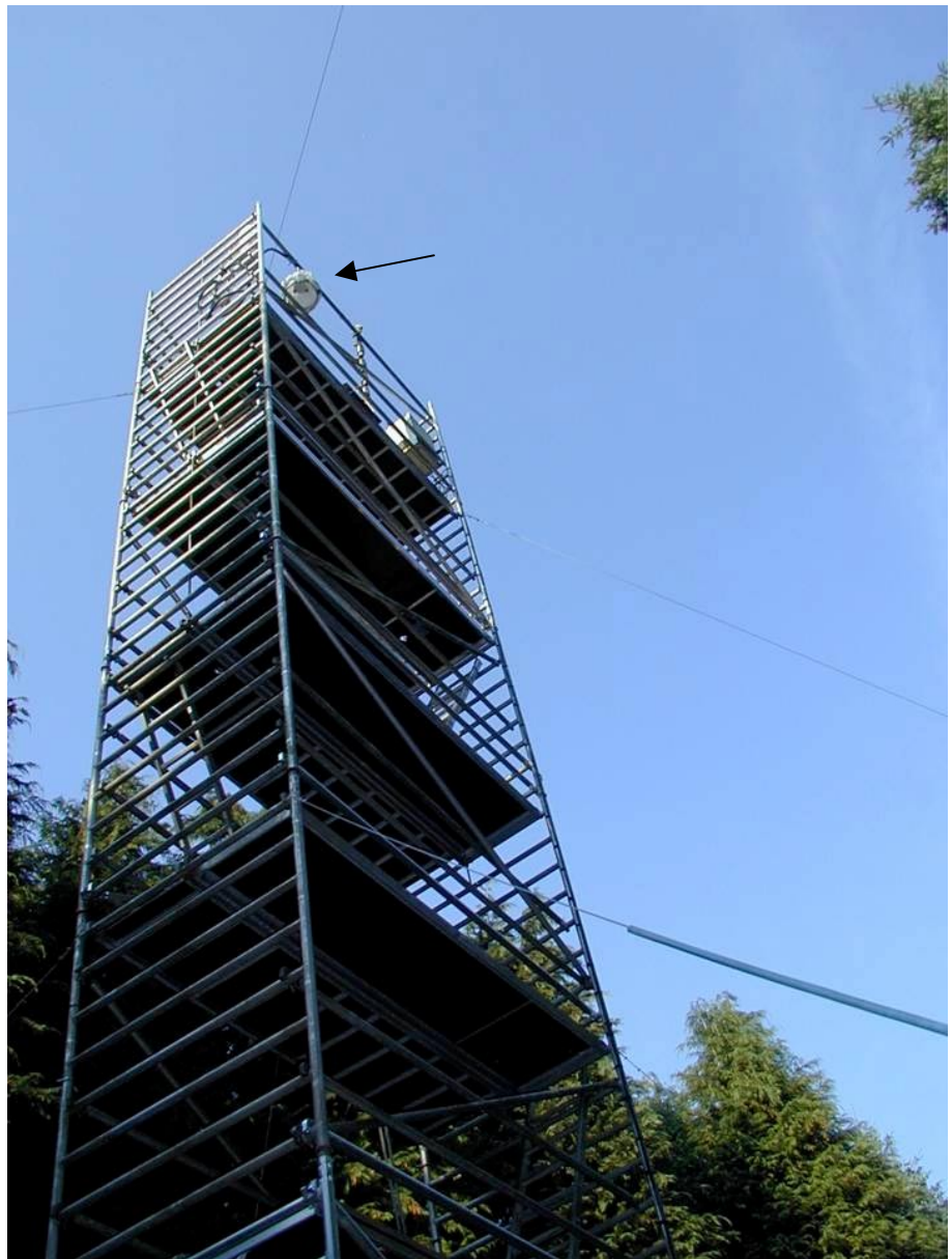
Figure 2. The 12 meter high scaffold in Frederiksborg. The rain protected air-intake is seen at the top
